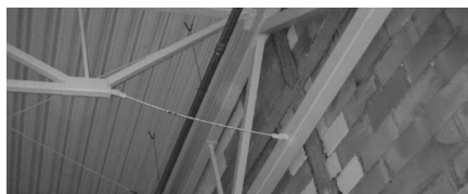
Fig. 4. Overextended strut due to improper prestress [29].
