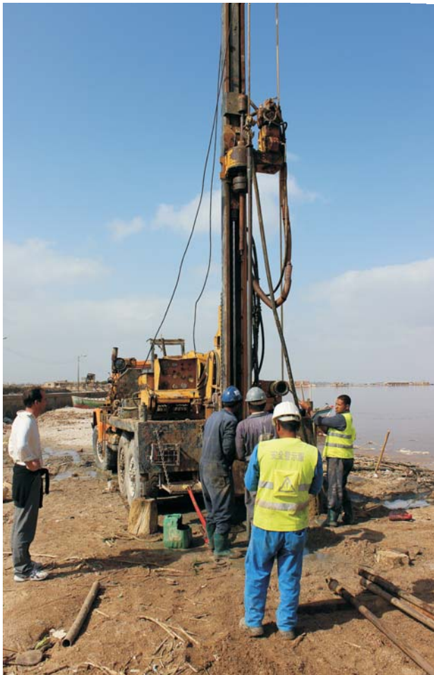
Fig. 3. Drilling FA-1 core in southern margin of the Qarun Lake, using a drilling rig of the Acer company.
